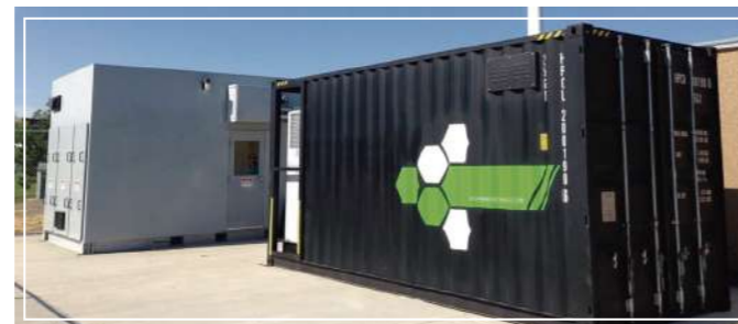
■ On-Grid Energy storage system
